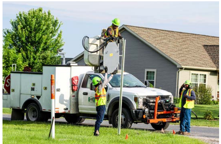
Webster Rd & Sarle Rd - Tittabawassee Twp Sign Shop / Replacement of Stop Sign
